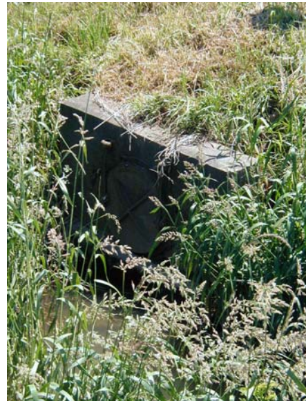
COMBINED SEWER OVERFLOW
