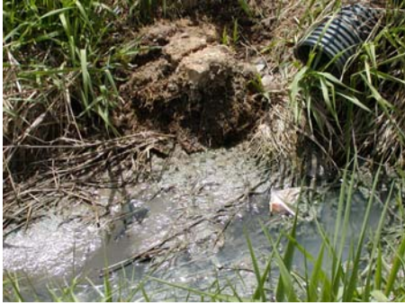
Discharge pipe from barnyard area
