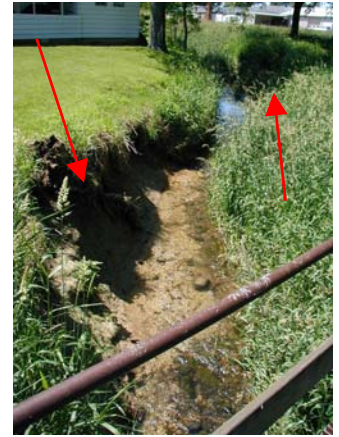
Erosion and bank sloughing along Werntz Ditch
