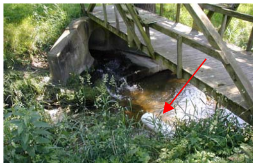
Discharge pipe with unknown source to Wertz Ditch
