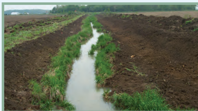
Figure 3. B: Modification of a ditch to a two-stage geometry by pulling the banks back to form benches.
