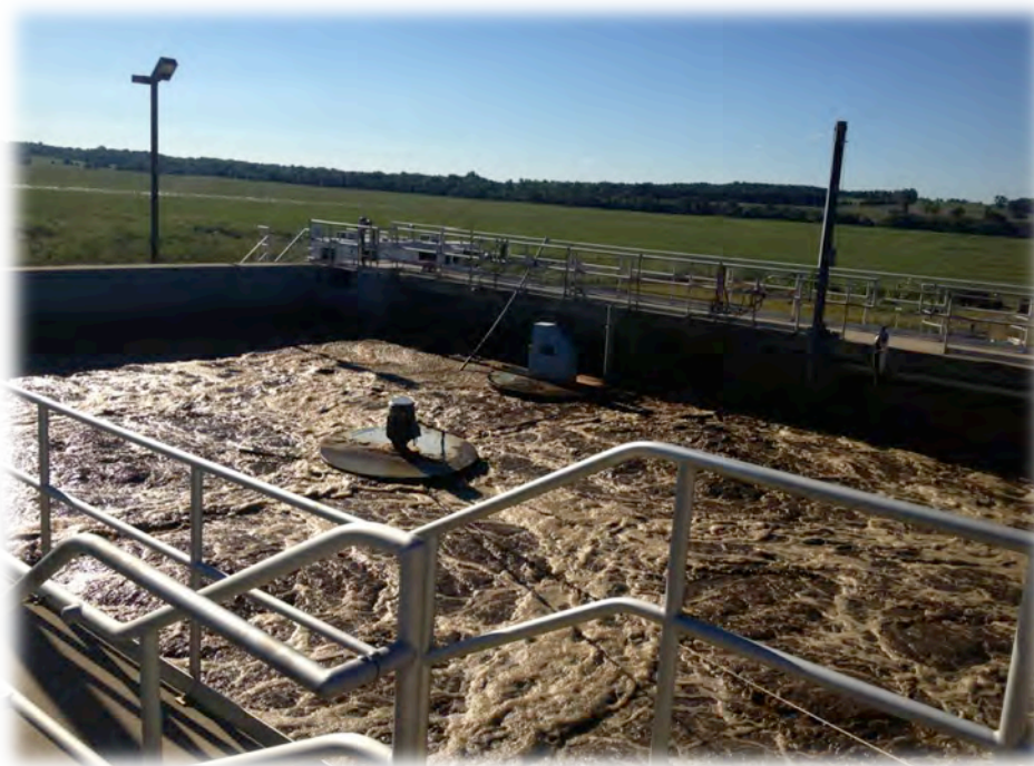
Steuben Lakes RWD Waste Water Treatment Plant
