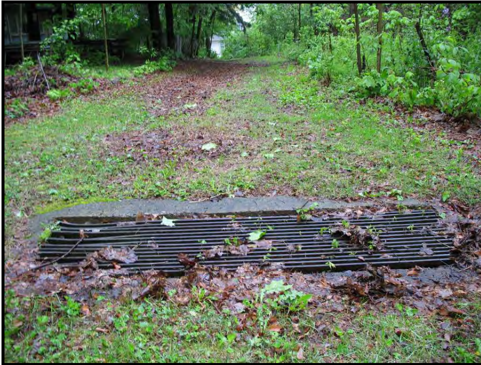
Figure 10.1. Metal grate covering 2x2 foot drain pipes.
