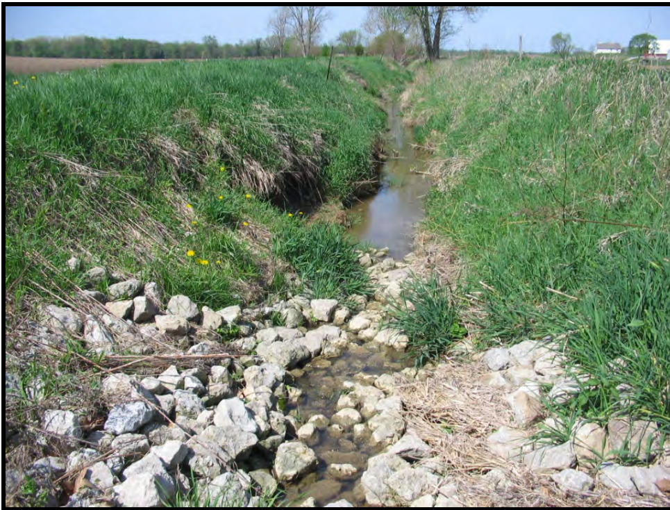
Grade control structure installed along Dillon Creek through the Watershed Land Treatment Program with the cooperation of the Noble County Surveyor's office.
