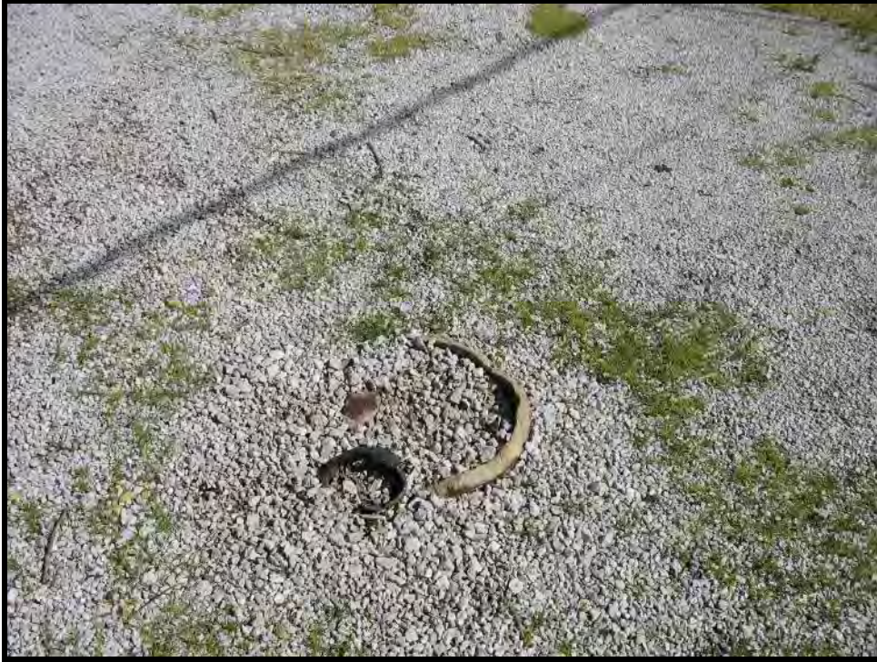
Figure 5.3. Gravel-filled storm drain.
