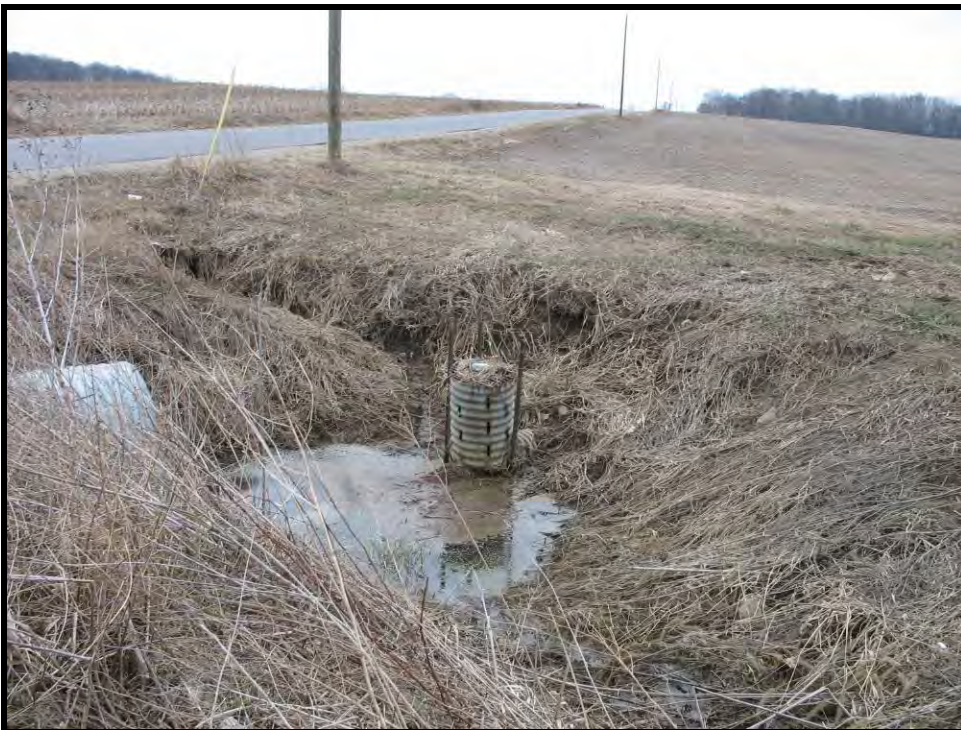
Erosion around tile lines in Dillon Creek Headwaters.
