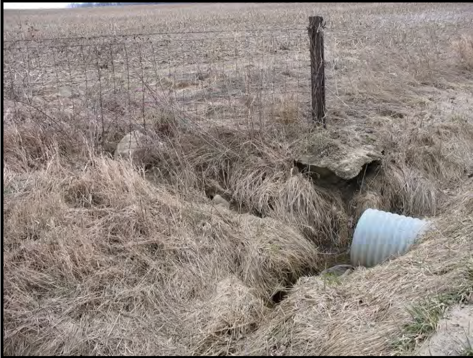
Erosion around tile lines in the Turkey Creek Headwaters.
