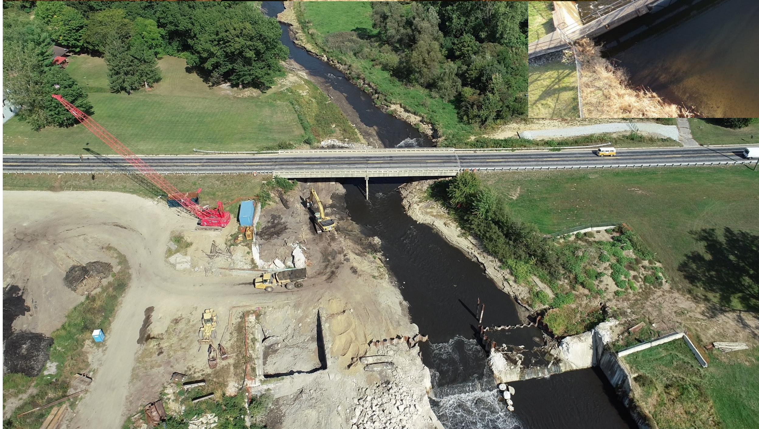
Dam removed slowly with coffer dams and a series of small drawdowns to lessen sediment movement downstream.
