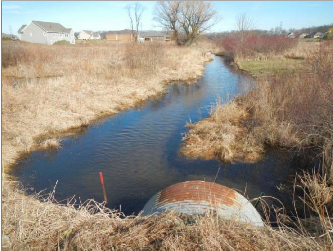
Perched culvert on Cobus @ CR 2
